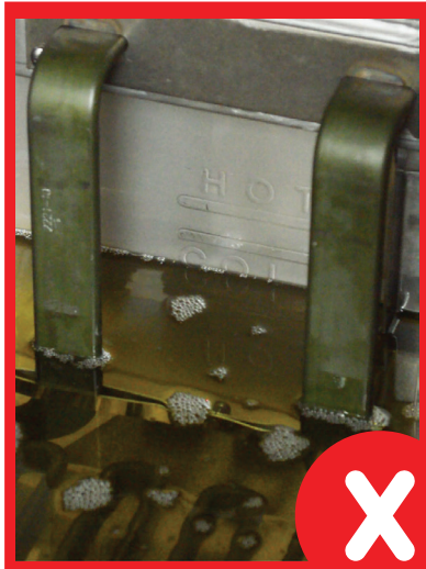
INCORRECT OIL LEVEL
